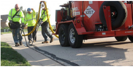
Crack sealing is a critical maintenance step; it helps the roadway combat water intrusion. (Image courtesy of Fahrner Asphalt Sealers)
